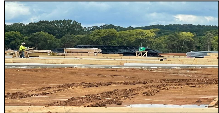
1.8 million square feet facility under construction less than 1 mile from site; just a sample of recently completed and under construction manufacturing and industrial in the area
